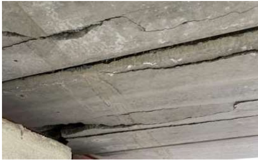
c) The area close to the support at right side after second impact
